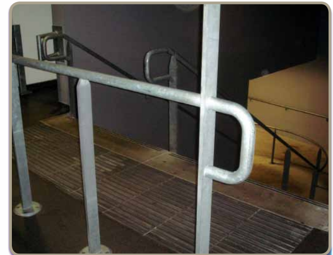
Figure 16 – Tactile paving (detectable warning) with a barrier at the top of the stairs
