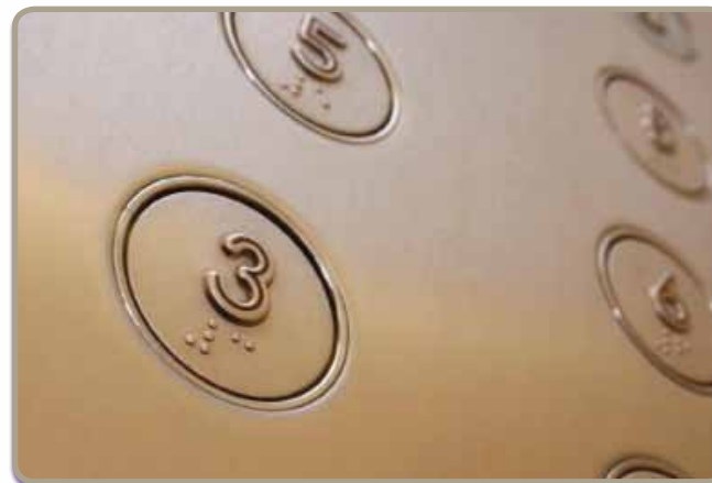
Figure 11 – A lift control panel with tactile and Braille symbols
